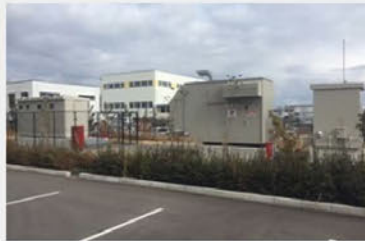
Emergency private power generation facilities
