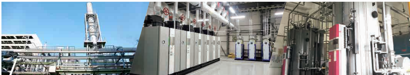
Otsuka Chemical: Cogeneration system at the Tokushima Factory Otsuka Pharmaceutical Factory: Boiler room at the Toyama Factory Otsuka Sims (Guangdong) Beverage: Gas boiler
