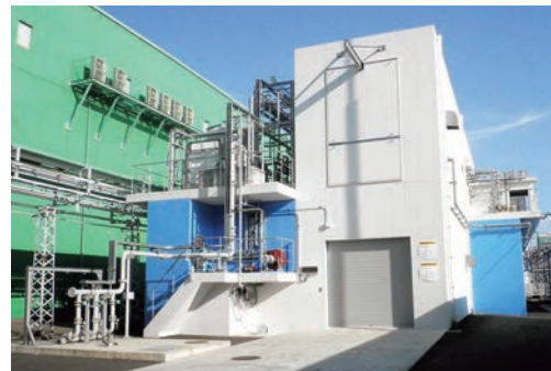
Otsuka Pharmaceutical Factory: Wastewater treatment facilities
