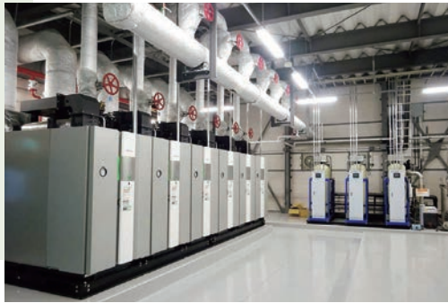
Otsuka Pharmaceutical Factory: Boiler room at the Toyama Factory
