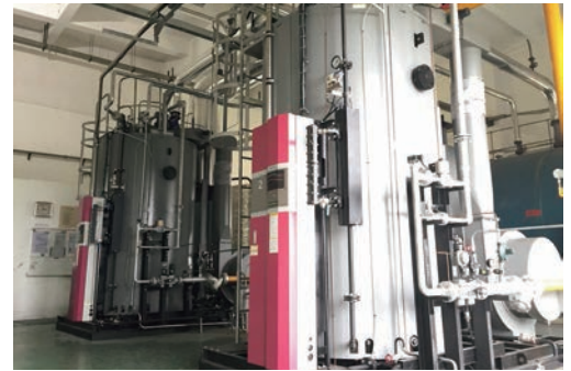
Otsuka Sims (Guangdong) Beverage: Gas boiler
