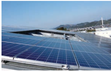
Solar power generation systems
