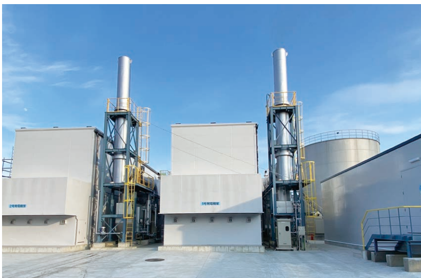
Otsuka Chemical's Tokushima Plant
